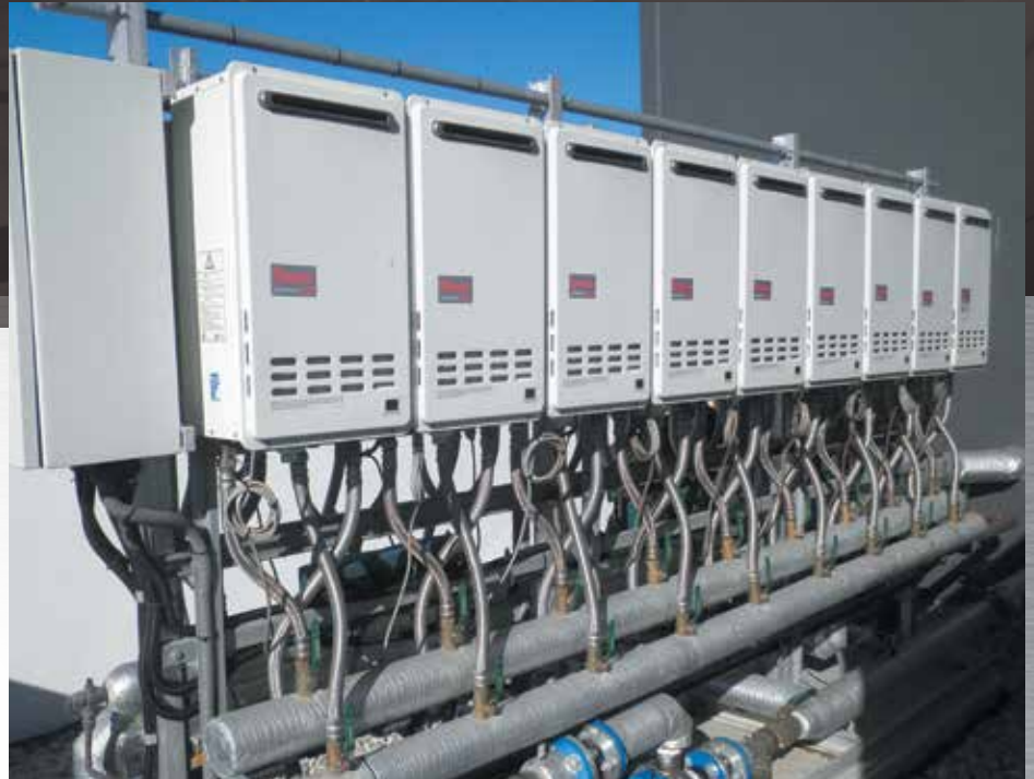
Photo: Back to back 18 Unit Commpak Plus®
