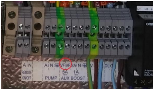
Picture of heat pump terminal strip
