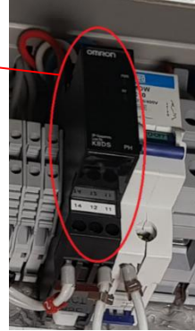
PHASE DETECT RELAY
