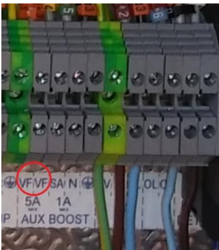
Picture of heat pump terminal strip showing VF connections
